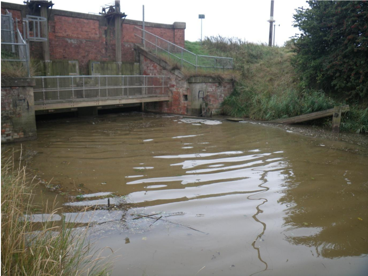
Plate 7. Sluice at Keyingham drain with visible surface ripples from estuarine water entering the drain at high tide.
